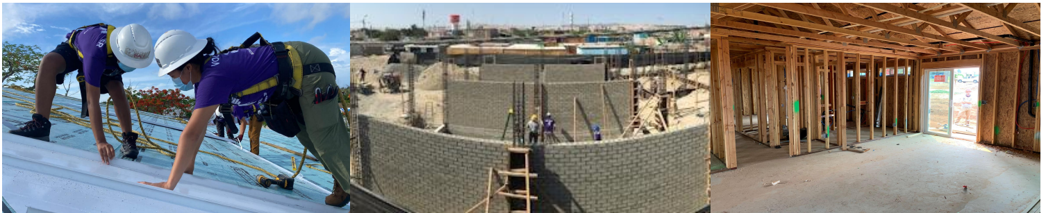
Photos: (L-R) Our team in The Bahamas working on the roof at ECC earlier this summer; Pre-COVID progress at Santa Cruz de Villacuri School; Early stage of one of our home rebuild projects in Northern California.
